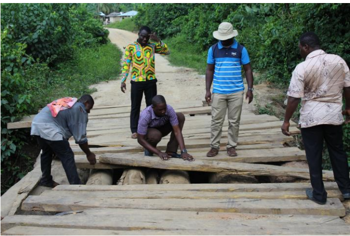
CSLP team repairing a bridge leading to one of the project intervention communities
