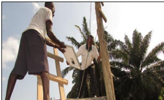
Figure 27 Solar Installation at Eshiem
