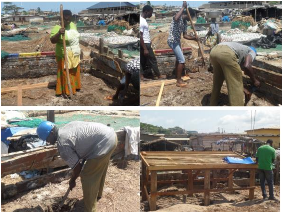
Figure 5: Some members of the association volunteered their time and effort during the construction of the raised racks in Apam in the Central Region of Ghana.
