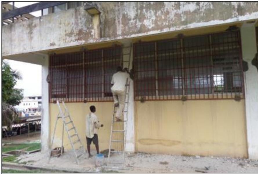
Figure 4 Town and Country Planning Department building and site of the Central Region Environmental Planning Data Hub Being Refurbished
