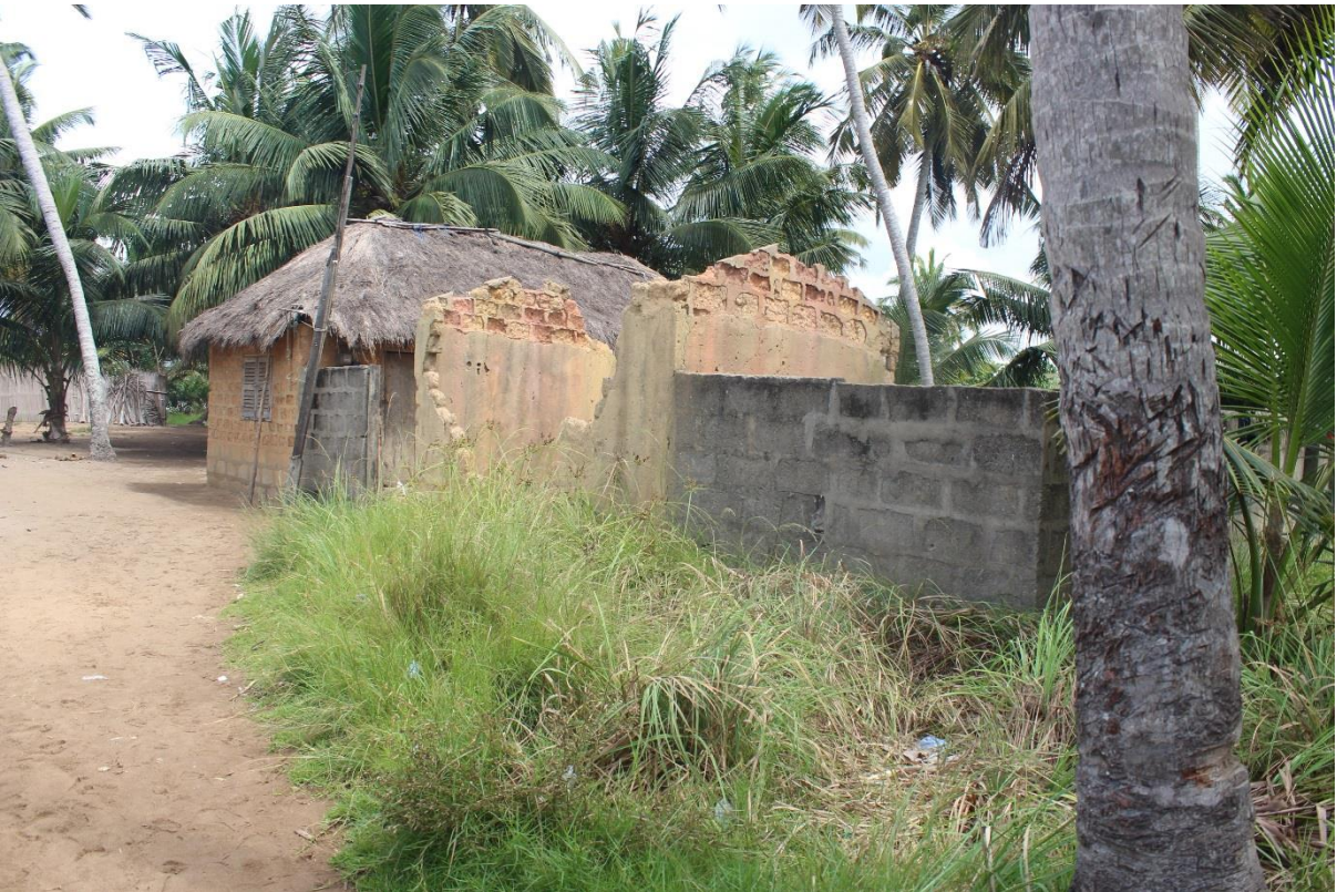
Figure 6 A collapsed structure due to effects of flooding
