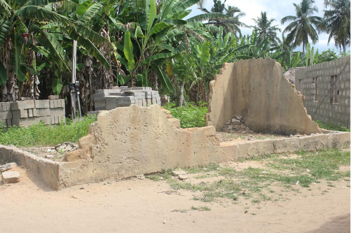
Figure 5 A collapsed structure due to effects of coastal erosion
