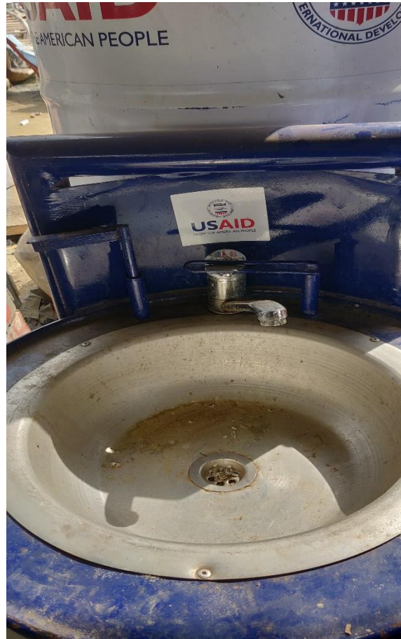
Figure 14 Broken down Handwashing station at Awudin
