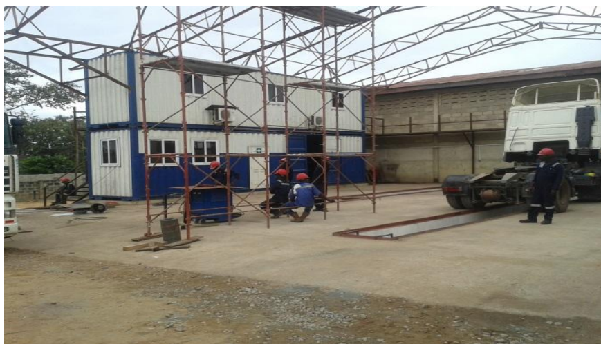
Safety harness and workers in their PPEs at the Baj Freight yard
