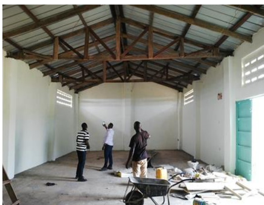
Nestle Procurement Manager inspecting the newly constructed warehouse 1 of Kha-ma Farms in Karaga in the Northern Region
