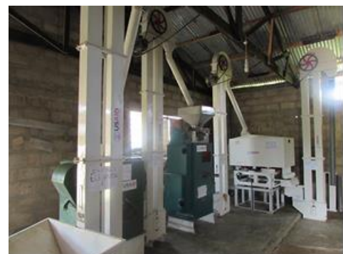
New rice mill installed for Sambay Enterprise of Bolga under grant
