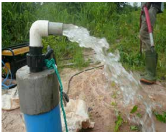
Picture 2. 4: Mr. Sarpong's Borehole and generator
