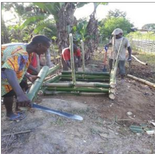
Figure 1. Using bamboo to construct a fence for the stockpile compost method at Adubrim.
