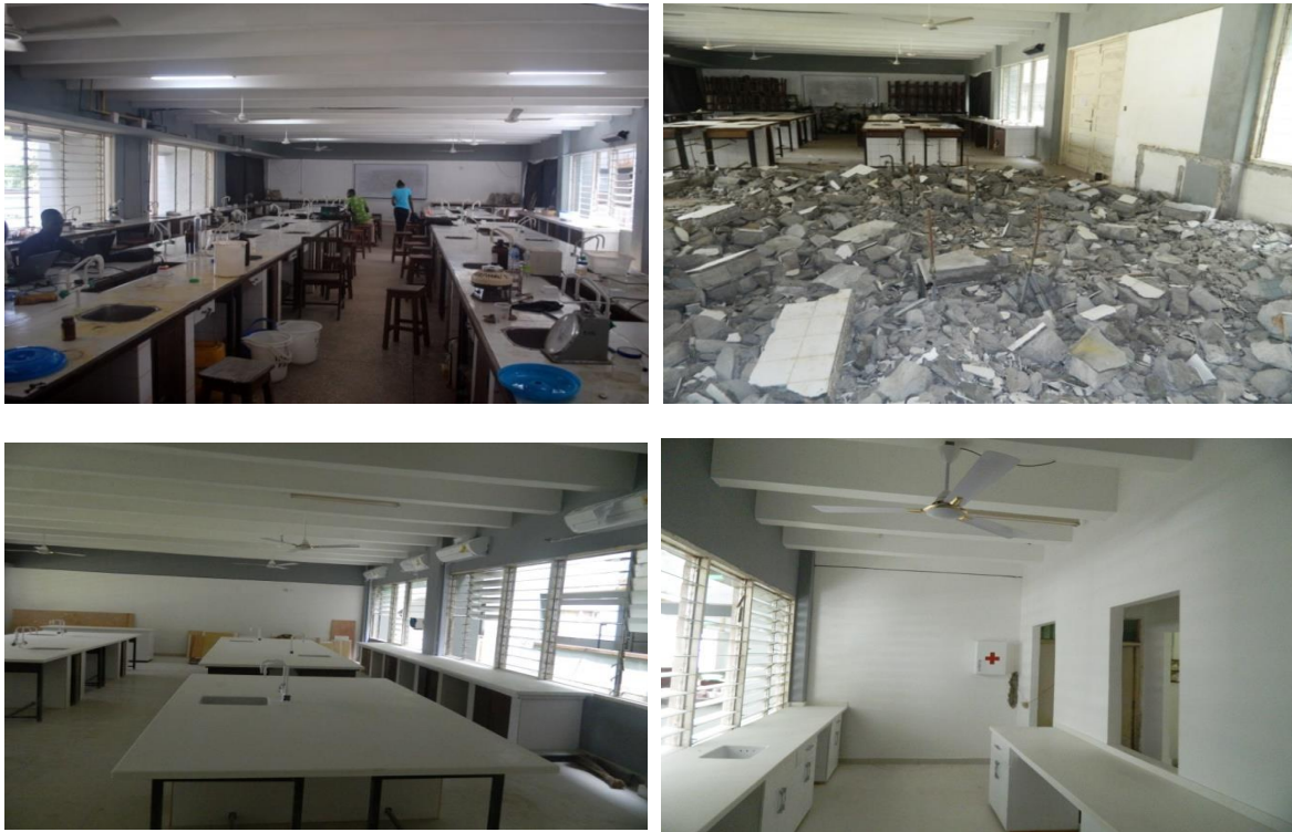
Figure 16: Fisheries and Coastal Research Laboratory before and during demolition works (Top) and current state of renovation (Bottom)
